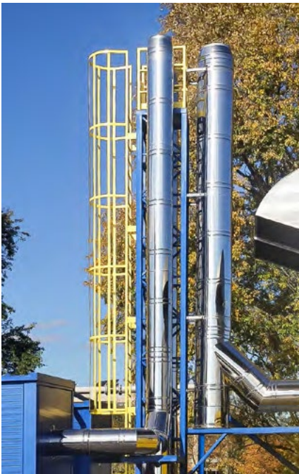
Small thermal power plant, Racibórz . Poland
